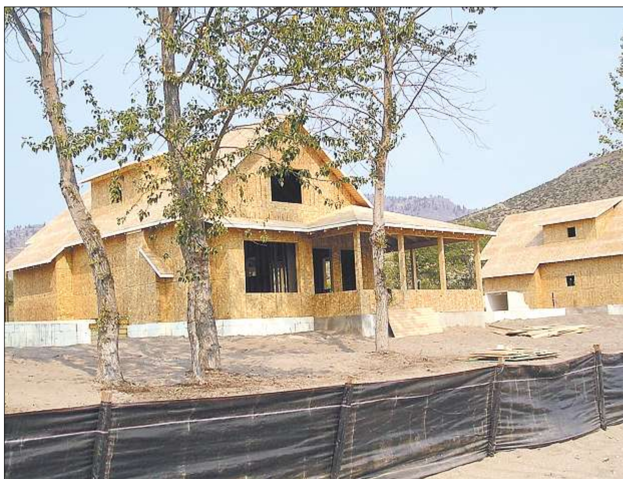
Veranda Beach under construction on the Washington state side of Lake Osoyoos by Legend Resorts. Courtesy, Peak Communicators
