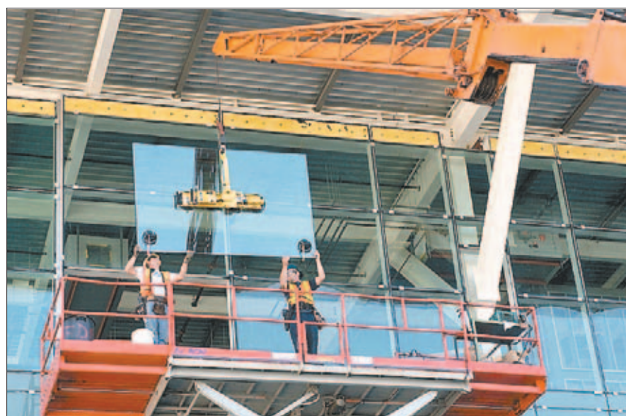
Construction workers install the last pane of glass for the expansion of the international terminal at Vancouver International Airport on Thursday.
